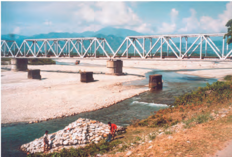
Photo 6. Remains of old bridge over Chel river dammaged during flood and replaced due to rising of channel floor, November 2007 (by L. Starkel)
