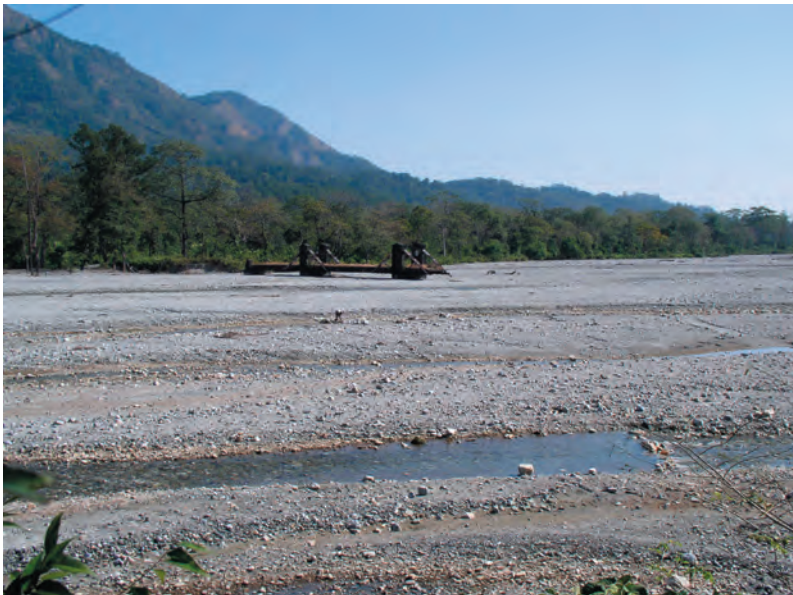
Photo 38. Braided channel in root part of alluvial fan of Jainti river with remains of bridge dammaged during flood in 1993 (by R. Soja)
