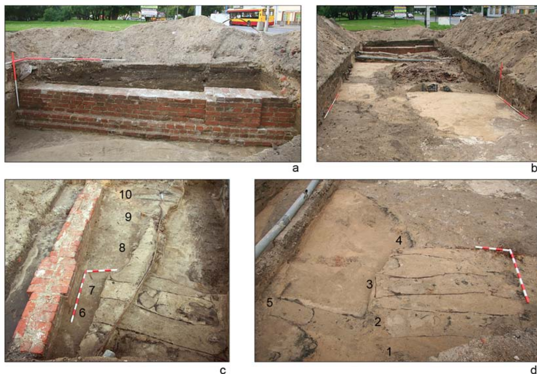
Fig. 5. Bródno Jewish Cemetery in Warsaw, archaeological excavations: a – trench 2, foundation of brick cemetery wall, view from the east; b – trench 2, location of waste pits and excavated fragments of matzevot ; c – trench 4, location of burial pits nos. 6–10; c – trench 4, location of burial pits nos. 1–5 and foundation of the cemetery wall. Photo: W. Bis.
