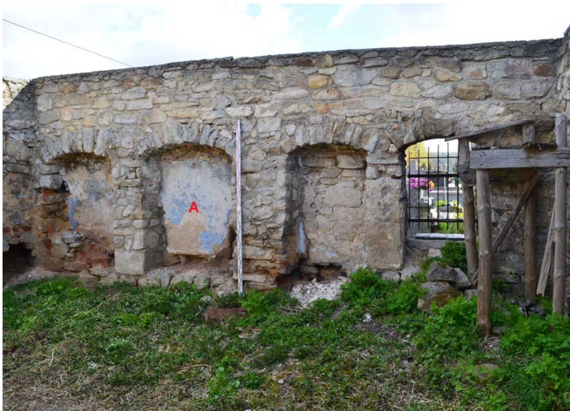
Fig. 16. Complex of the Holy Spirit in Szydłów, the north hospital wing, east wall of the patient's room: A – Former doorway to the latrine, 2017. Photo: M. Cichocki.
