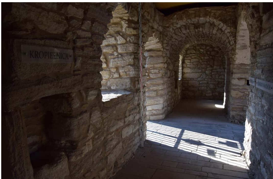
Fig. 12. Complex of the Holy Spirit in Szydłów, the western corridor of the ambulatory porch from the south side. Condition after conservation, 2025. Photo: T. Olszacki.
