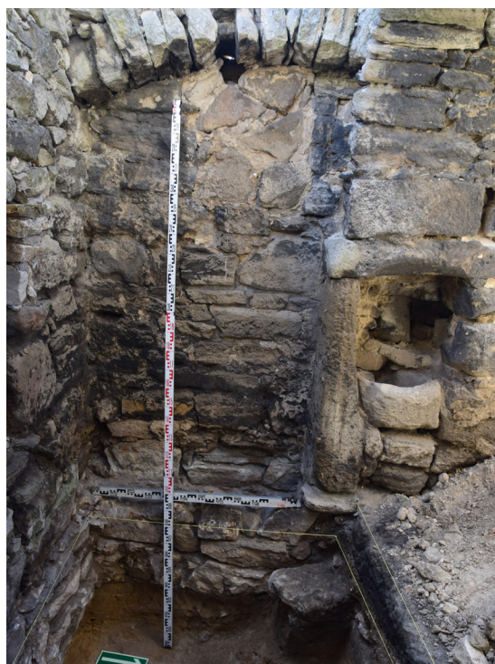
Fig. 13. Complex of the Holy Spirit in Szydłów, the archaeological excavation 7/2017: corner of the hospital's southern wing and the western corridor of the ambulatory porch with stoup (Phase Four) introduced into the north part of the niche of the Phase Three, 2018. Photo: T. Olszacki.
