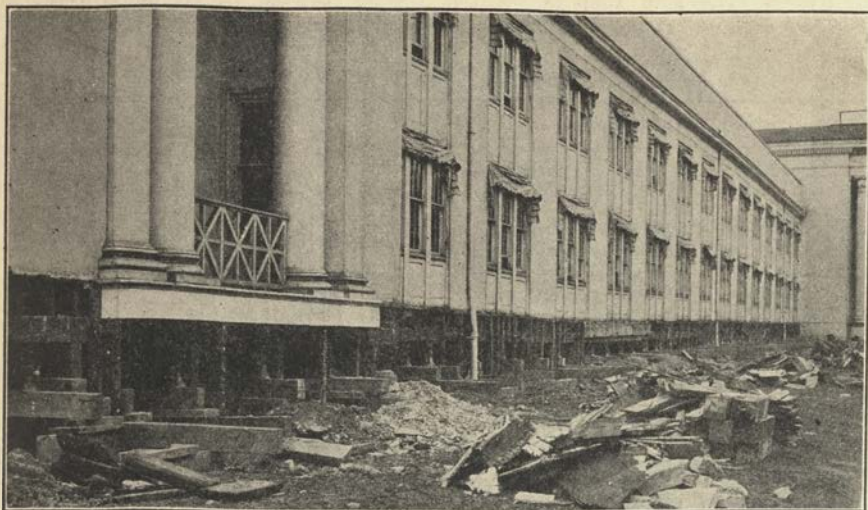
Fig. 15.—A public building, the foundation timbers of which have been badly damaged by termites, necessitating extensive repair work. (From photo by Snyder, U.S.D.A.)
