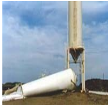
Figure A.2. Failure of grain silo.
