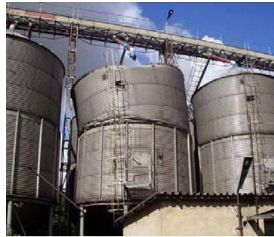
Figure A.4. Failure of grain silo, 2005, Brzeg, Poland, (implosion).
